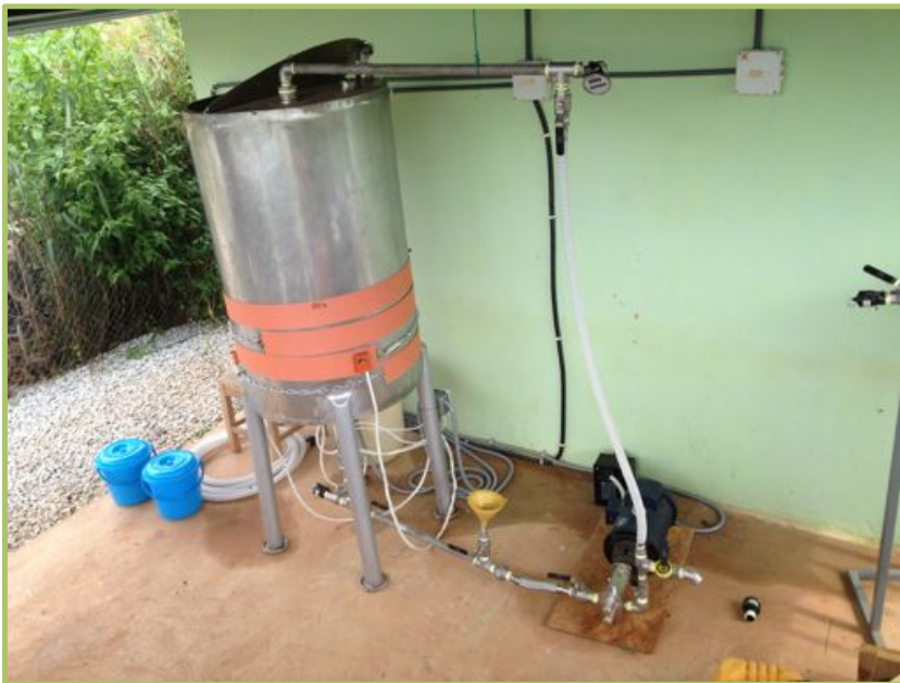
The imperfect biodiesel tank...note the puddle on the floor.
